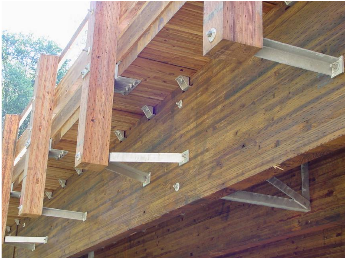
Photo 1. Timber Bridge with aluminum deck clips.
