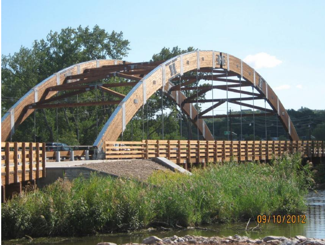
Photo 2. Overpeck Park Bridges in Teaneck, New Jersey are designed to carry two lanes of traffic with HS25 loading.
