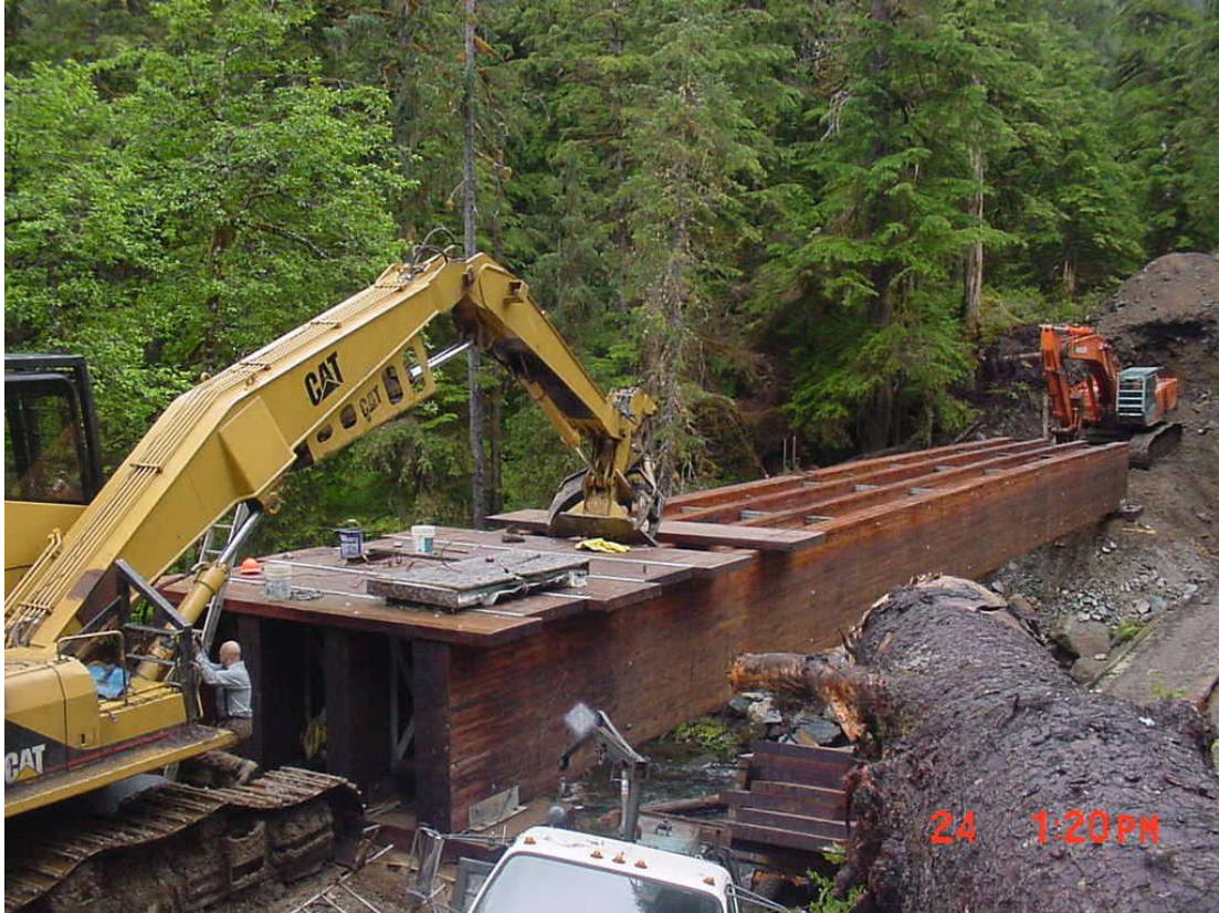
Photo 6. Alaska Logging Bridge using backhoes for installation. (Photo Courtesy of Eleanor Oman, US Forest Service)
