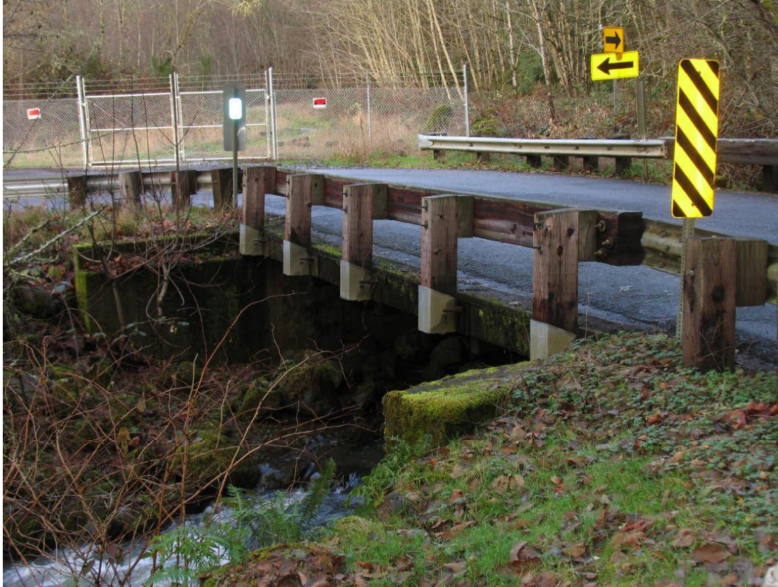
Photo 4. A timber longitudinal deck bridge with a TL-2 rail without a curb.
